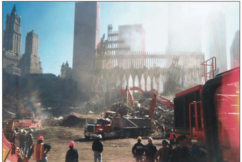
A Truck Receiving a Load of Debris for Removal from the World Trade Center Disaster Site.
